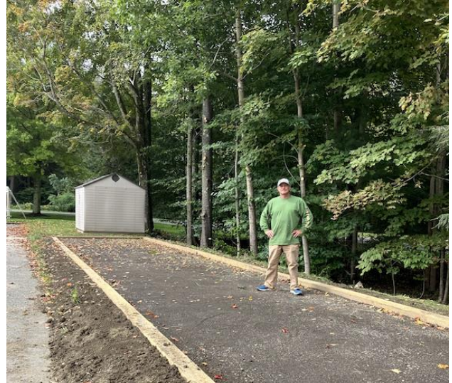
Grounds Supervisor Derek Powell stands on leveled surface of the new bocce court that awaits installation of artificial turf.
